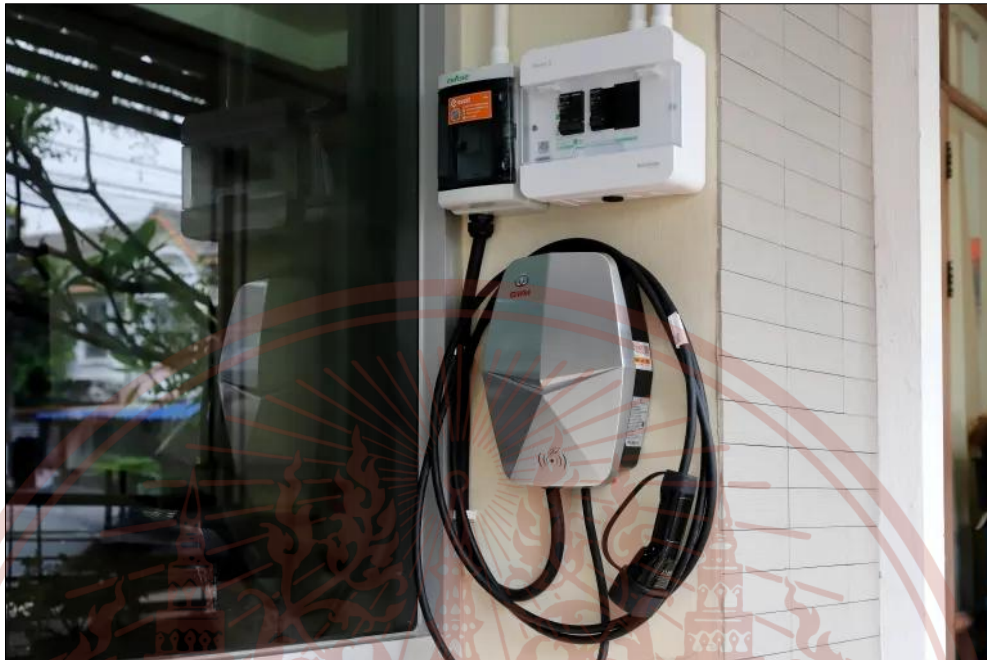
Figure 2-8 Home electric car charging equipment (Chaidee, 2023)
